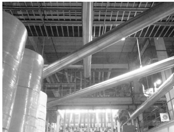
Figure 17: Existing Pipe Lines and Wire Trays
