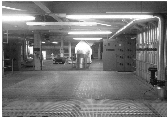
Figure 15: Air Heaters Area
