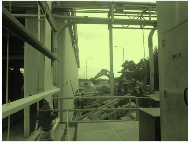
Figure 14: New Compressor Area
